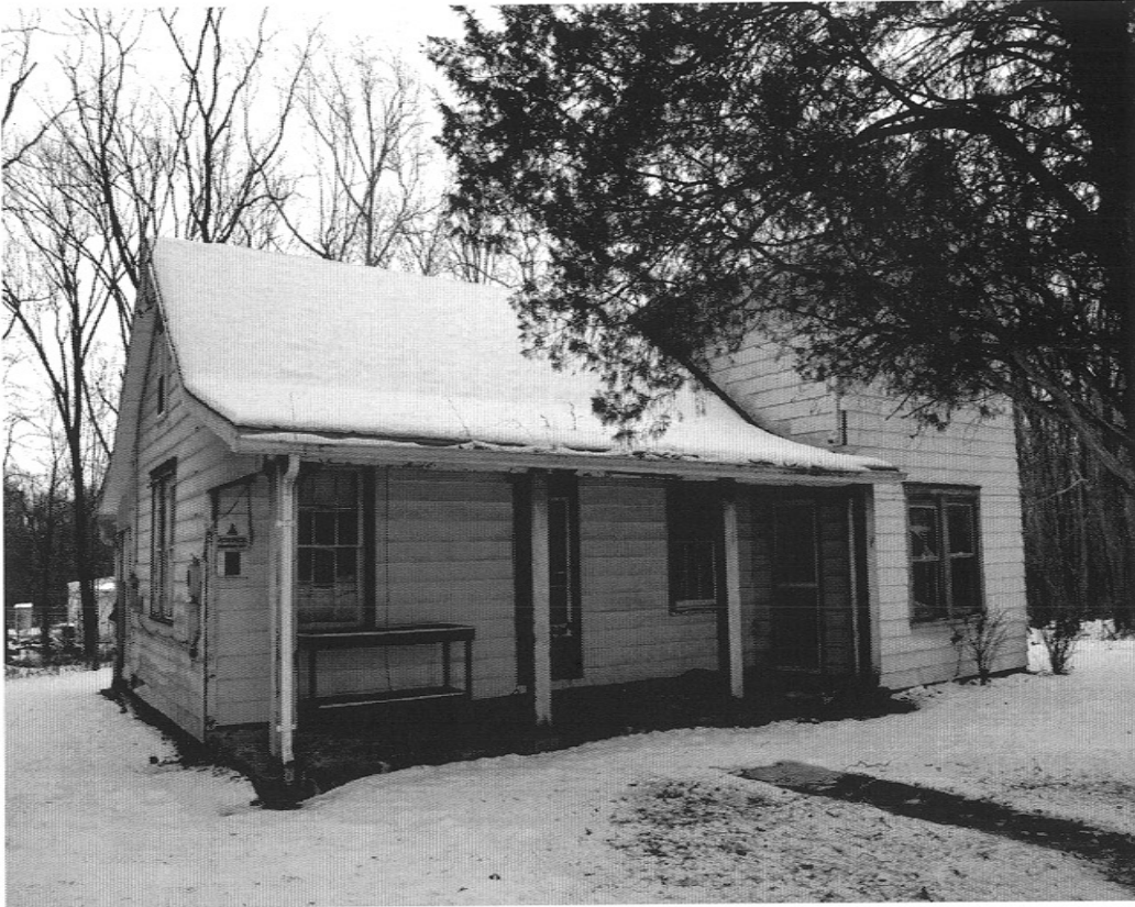
The Fort Frederick Colored Schoolhouse, or the Williams Schoolhouse as it is also known, survives despite later alterations, including the porch and two-story addition at right.
