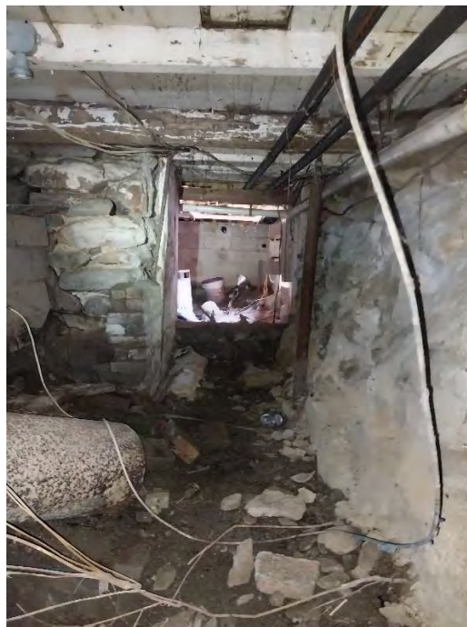
Figure 73: Crawl space entrance from within the crawl space, looking into the cellar area. As can be seen, it was difficult to distinguish the stone hearth base (left) from the rest of the stone foundation before excavation. (11 August 2023). Image courtesy of David Bittle.
