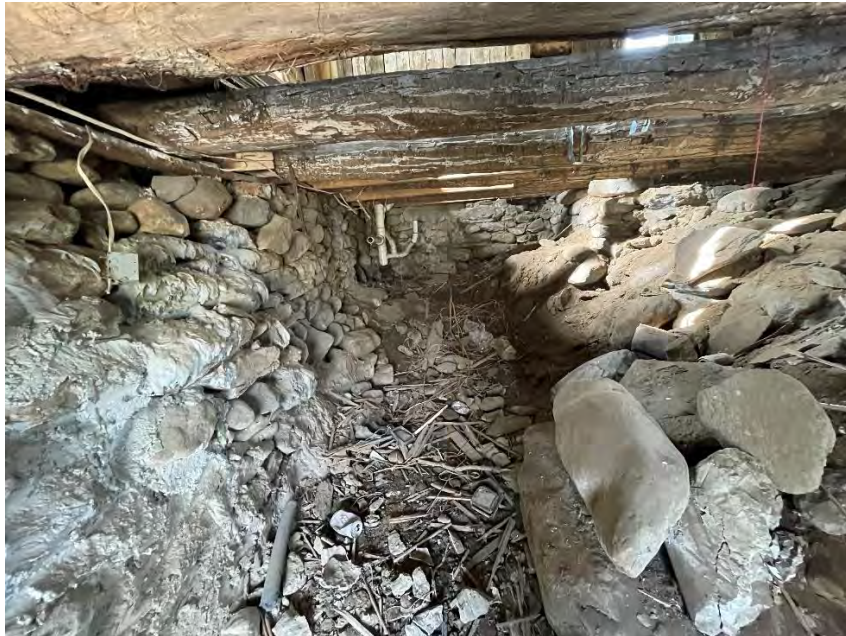
Figure 25: Crawl space beneath the original dwelling post-excavation. The original log floor joists and stone foundation walls are all in full view. The stone wall blocking access to the eastern portion of the crawl space can also be seen to the right, rising from the ground to the floor joists. (25 April 2024).
