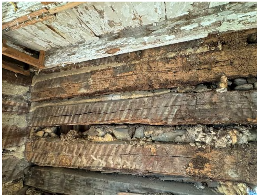
Figure 81: Close-up of the interior north wall post-excavation, with a more detailed view of the original horizontal logs and the chinking between them. (10 September 2024). Image courtesy of Elizabeth Comer.
