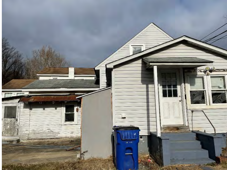
Figure 34: Hoke dwelling from the south. The south addition, with its covered doorway, double window, and gable frame asphalt shingle roof are in the foreground. To the left is the west addition with the summer kitchen and anteroom. The summer kitchen's south window, gable frame asphalt shingle roof, and metal overhang with wooden pole rafters are all visible, as is the anteroom's lean-to roof and screen door. Also to the left are the concrete patio and lean-to structure attached to the south addition.
