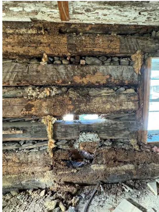
Figure 83: Gap in the horizontal log wall where the gas heating system was installed around the center of the original structure's north elevation. More of the chinking between the logs is also visible, much of which appears to be composed of wood and stones. The north elevation window is also in view to the right. (10 September 2024). Image courtesy of Elizabeth Comer.
