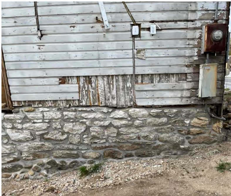
Figure 61: Section of the original vertical board siding revealed by the excavation, as well as the wood Dutch lap siding covering it. (25 April 2024).
