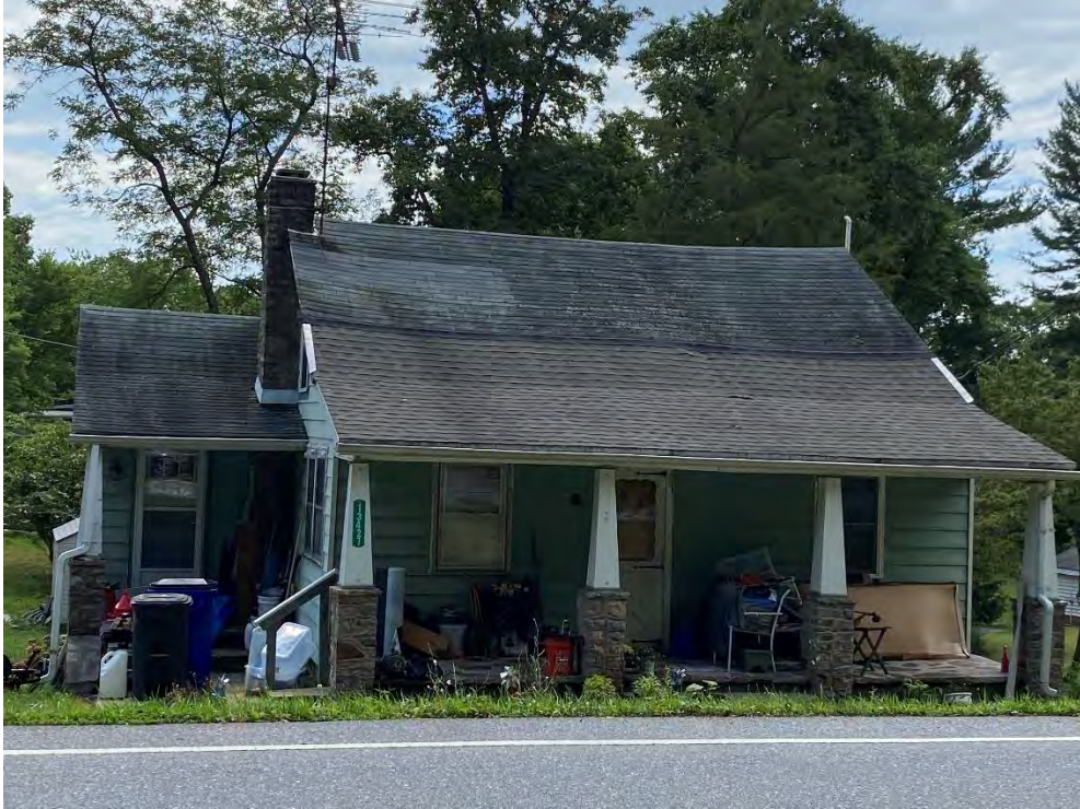
Figure 2: 13427 Catoctin Furnace Road at the northern edge of Mine Bank, still retaining its fundamental design akin to the other early 19 th century Catoctin Furnace worker homes. Image courtesy of Elizabeth Comer.
