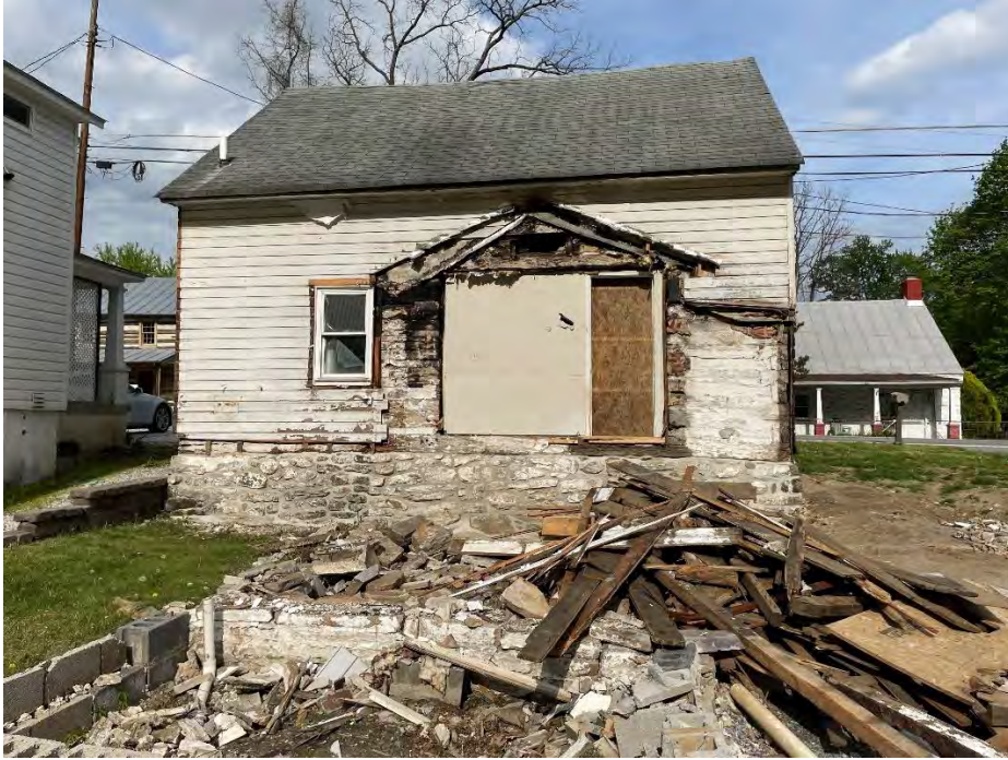
Figure 14: Post-excavation photograph of the Hoke dwelling west elevation, revealing sections of the original stone foundation and log siding. The outlines of the west addition and outdoor tool closet can both be seen on the dwelling, as well as the doorway that once connected the west addition with the main structure. The restroom window, as well as remains of the west addition's stone and brick foundation, are also extant. (25 April 2024).
