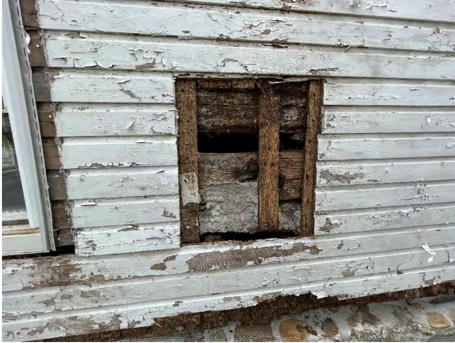
Figure 68: Exterior view of the hole where the Smith family installed the gas heating system into the north elevation wall in 1979. The hole was cut into the previous wood Dutch lap siding, hidden beneath the modern vinyl siding until the 2024 excavation. The hole provides a view of the dwelling's original vertical board over log construction. (25 April 2024).
