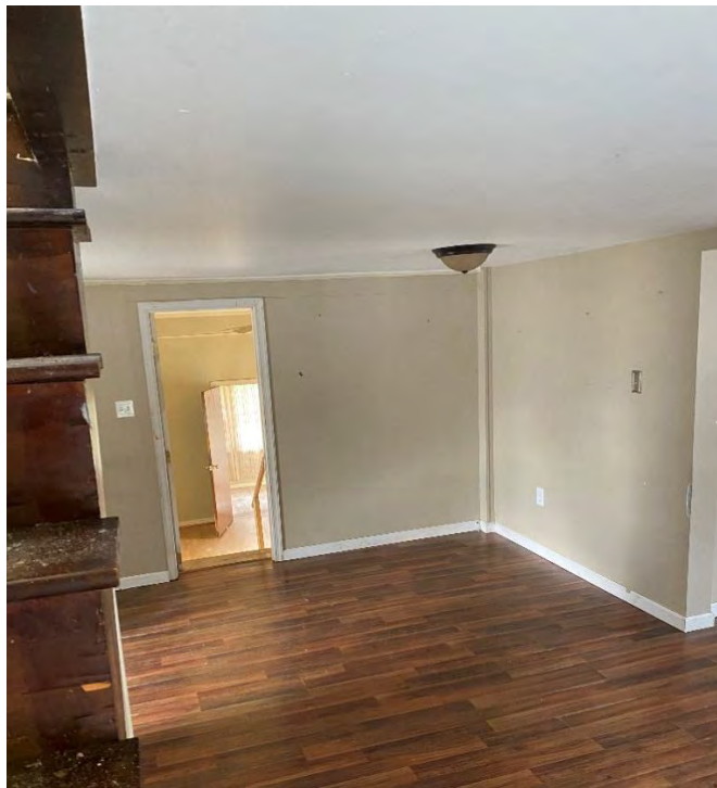
Figure 17: Entrance to the west addition from the living room staircase, providing a view of the southwest section of the living room, and of the doorway's proximity from the boxed header at the far right. The summer kitchen and anteroom doorway can also be seen. (19 December 2023). Photograph by Elizabeth Comer.
