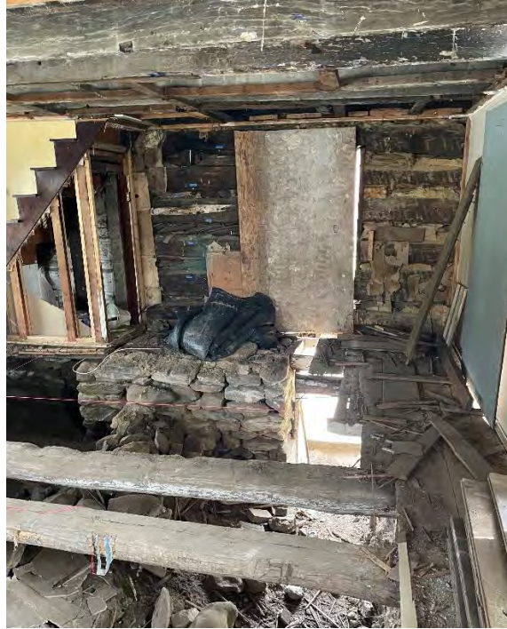
Figure 72: Southwest elevation of the original dwelling interior post-excavation from what was once the restroom. Image provides a full view of the stone base of the dwelling's original hearth and chimney, along with the original log and wood board wall and the former cased opening on the south elevation of the dwelling. Also in view are the crawl space entrance and original wood floor joists. (25 April 2024).
