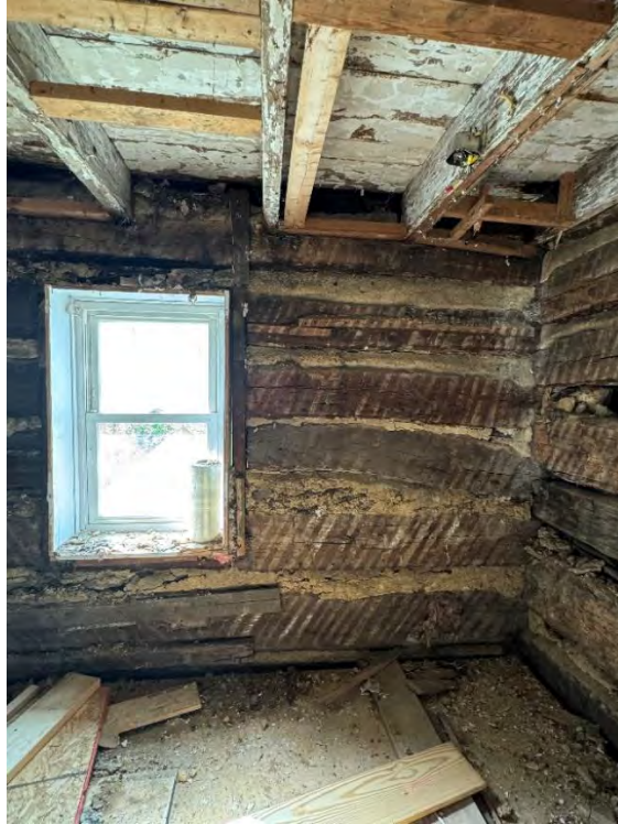
Figure 84: Northern section of the west elevation interior wall post-excavation, showing the west elevation window, the wooden ceiling and floors, and the horizontal log walls. The chinking in this area of the wall appears to be made from a much more uniform composition of materials than on the north elevation. (10 September 2024). Image courtesy of Elizabeth Comer.
