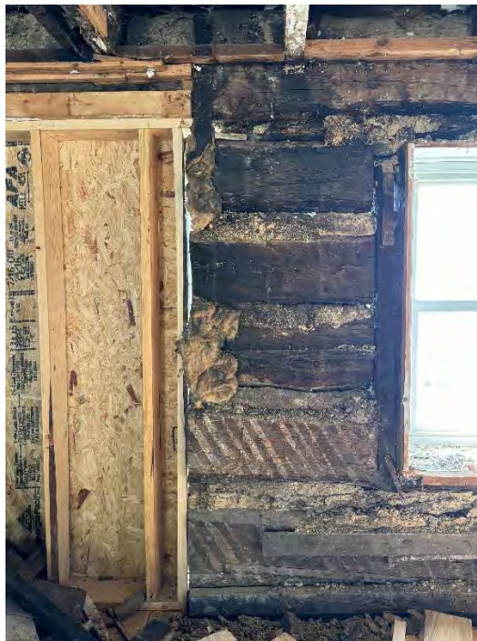
Figure 91: Post-excavation view of the west elevation interior log wall between the entrance to the since removed west elevation and the former bathroom window. (10 September 2024). Image courtesy of Elizabeth Comer.
