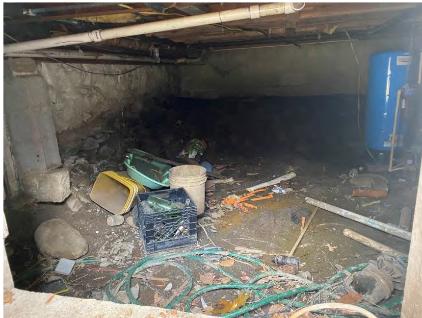
Figure 41: Shallow cellar area beneath the south addition, with a view of the CMU foundation wall and the north original stone foundation left of it. The dwelling's water tank is visible to the right. The moisture seeping out of the earthen floor of the cellar can also be seen, demonstrating the excess groundwater in the area.
