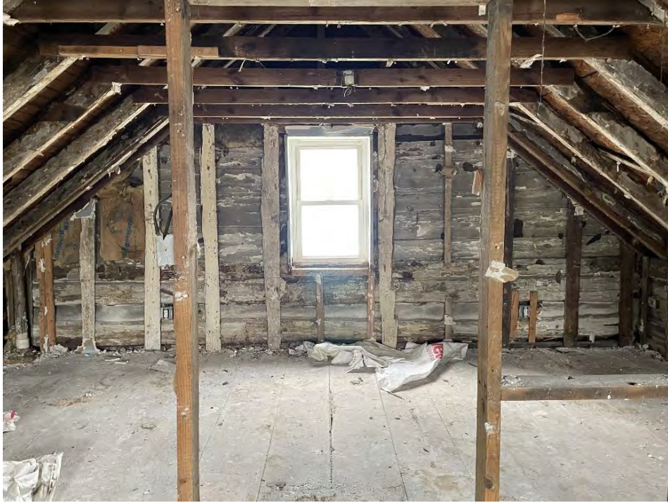
Figure 62: Original second-story horizontal wood board walls seen from within the dwelling. (25 April 2024).
