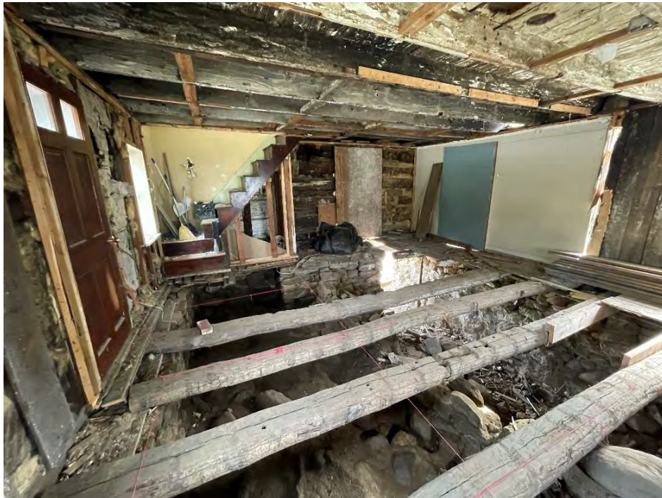
Figure 29: Wide view of the living room post-excavation, depicting many of the extant original components of the dwelling structure, alongside the nonoriginal stairs and front door. The sections of drywall that have not yet been removed are visible along the staircase and the former west addition entrance. The covered entrances to both additions are also visible. (25 April 2024).
