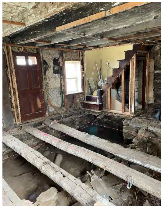
Figure 65: Southeast elevation of the living room post-excavation, depicting the original log floor joists and stone foundation, as well as the frame surrounding the front window, which once housed the front door. The bottom step of the staircase is directly against the old doorframe, indicating why the front door was moved. The original stone foundation along the east and southeast sides of the dwelling can also be seen. (25 April 2024).
