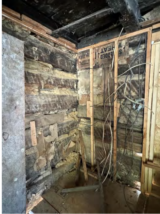
Figure 90: Southwest corner of the original dwelling post-excavation, displaying the covered entrances to the since removed south (left) and west (right) additions, along with the original log walls between them. Once again, the chinking between the logs in this part of the dwelling is much more uniform than that on the north elevation. The wood ceiling can be seen noticeably blackened at the top of the image, quite likely due to charring from the large house fire on 15 December 1979. (10 September 2024). Image courtesy of Elizabeth Comer.
