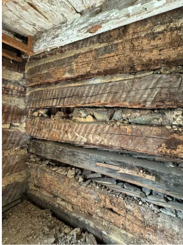
Figure 80: West corner of the original structure's north elevation wall after the vertical wood plank wall (see Figure 27) had been removed, showing the original horizontal log construction and part of the original wood ceiling. The chinking between the logs and the various materials it is composed of are clearly visible. (10 September 2024). Image courtesy of Elizabeth Comer.
