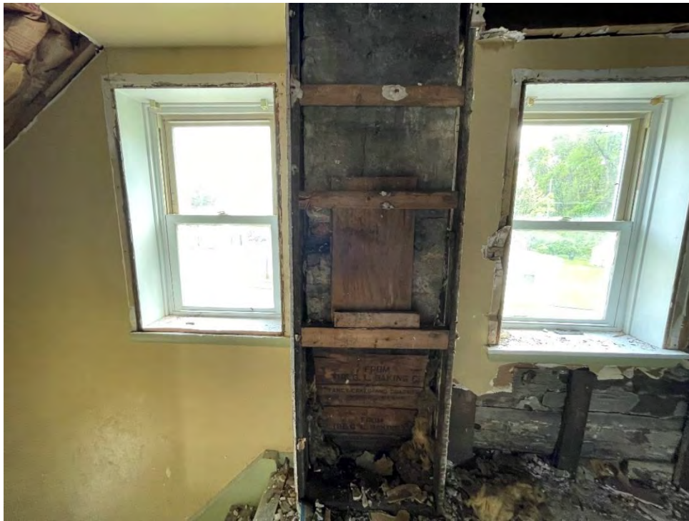
Figure 69: Post-excavation image of the stone brick chimney stack and two crates that were concealed behind the second-story bump out. (25 April 2024).
