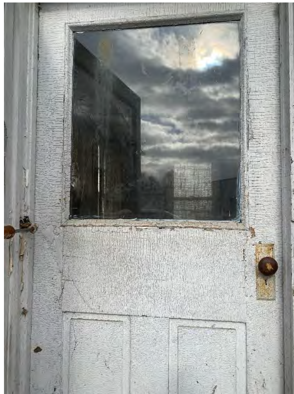
Figure 37: Windowed anteroom door exiting onto the rear patio. (19 December 2023). Photograph by Elizabeth Comer.
