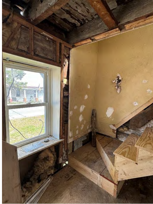
Figure 88: Southeast corner of the original structure post-excavation, showing the southern front window and newly rebuilt staircase, as well as the plywood covering the original log wall. The original wood in the ceiling is also visible at the top. (10 September 2024). Image courtesy of Elizabeth Comer.
