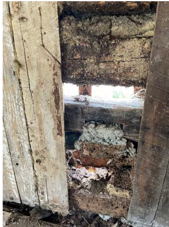
Figure 67: Interior view of the section of wall where the Smith family installed the gas heating system in 1979. The dwelling's original vertical board over log construction can be seen via the hole in the wall. (25 April 2024).
