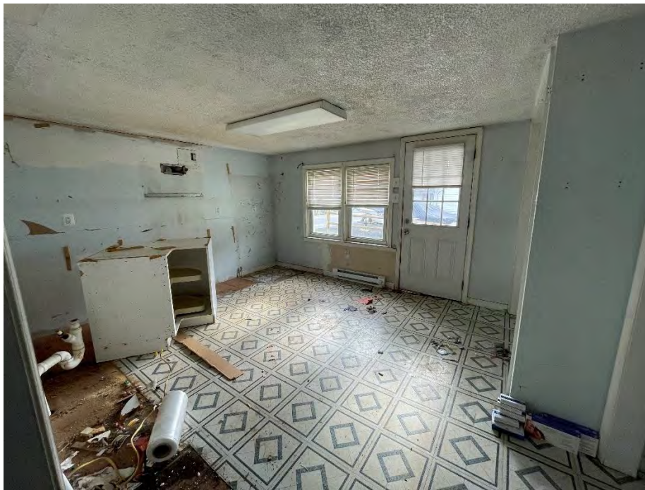
Figure 39: Kitchen from the cased opening, showing the door leading onto the driveway, the double window, and the peel and stick tile flooring.
