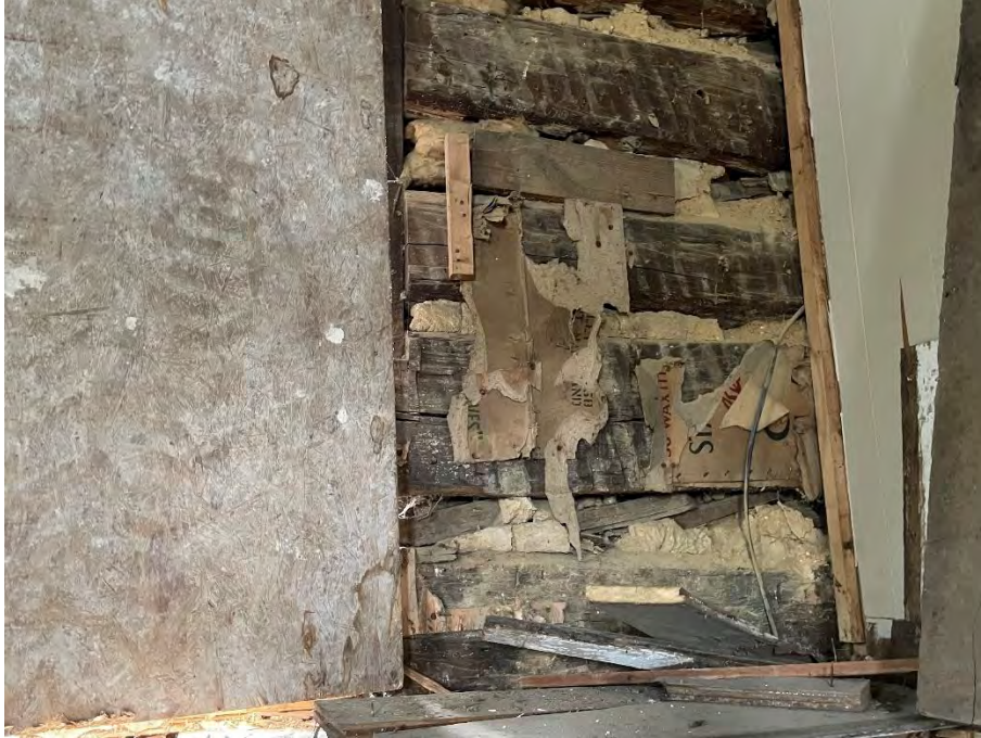
Figure 30: Interior remnants of poster paper used as insulation attached to the original log wall in the southwest corner of the dwelling structure. The chinking (sealant material used to fill gaps between logs in log buildings) between the logs is also visible. (25 April 2024).
