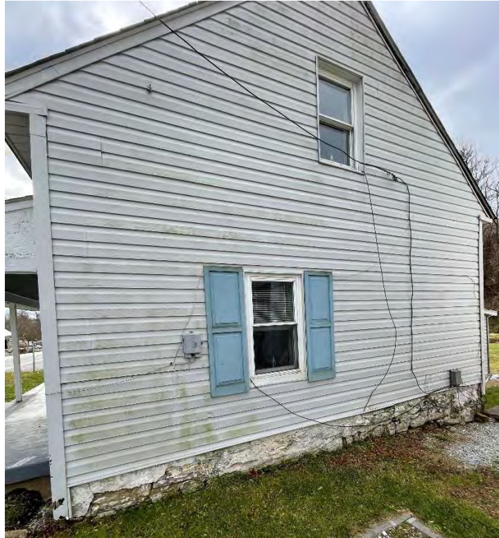
Figure 10: North elevation of the Hoke dwelling, showing the different positioning of the first- and second-story windows, as well as a portion of the dwelling's original stone foundation.
