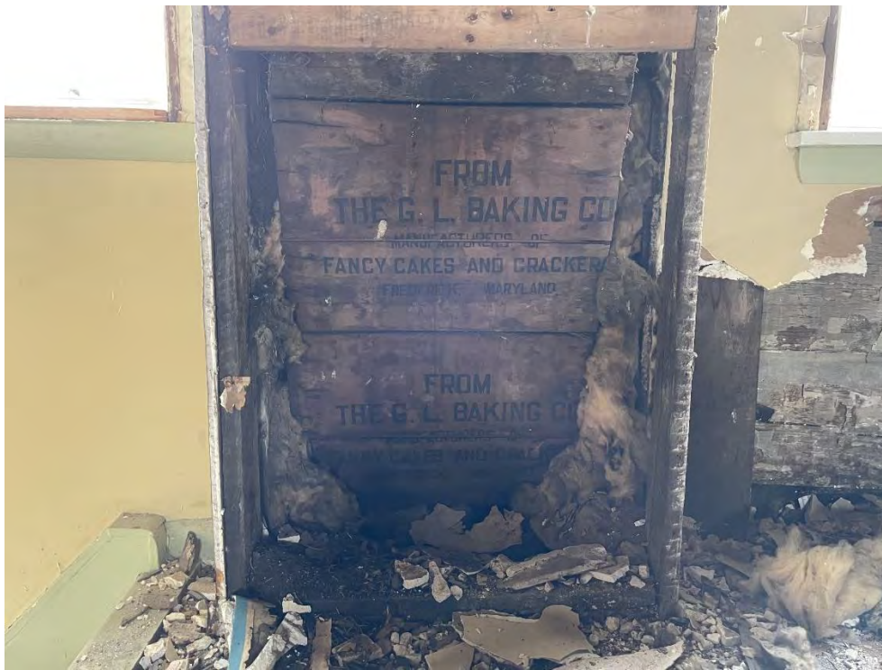
Figure 71: Crate fragments wedged beneath the chimney stack. The words "FROM THE G. L. BAKING CO. MANUFACTURERS OF FANCY CAKES AND CRACKERS FREDERICK, MARYLAND" can be seen on both crates. (25 April 2024).
