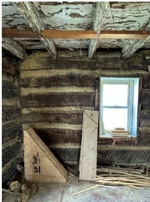
Figure 85: Northern section of the east elevation interior wall post-excavation showing the northernmost east elevation window and more of the wooden ceiling, floors, log walls. Like the northern west elevation, the chinking in this area of the wall appears to be made from a more uniform composition of materials. (10 September 2024). Image courtesy of Elizabeth Comer.
