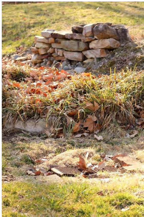
Figure 57: Rusted grate in the Carty-Miller rear yard. (5 March 2023).
