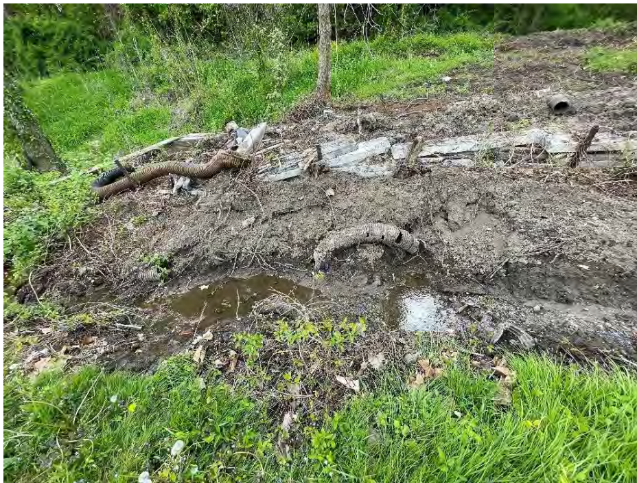
Figure 49: Section of the trolley bed hill post-excavation. Most of the brush has been removed, revealing the concrete slab wall and the disarticulated plastic culvert pipes. Flowing along the hill is water from the rusted grate in the Carty-Miller rear yard, which was temporarily uncovered when the stream pipe was ruptured in 2024. (25 April 2024).
