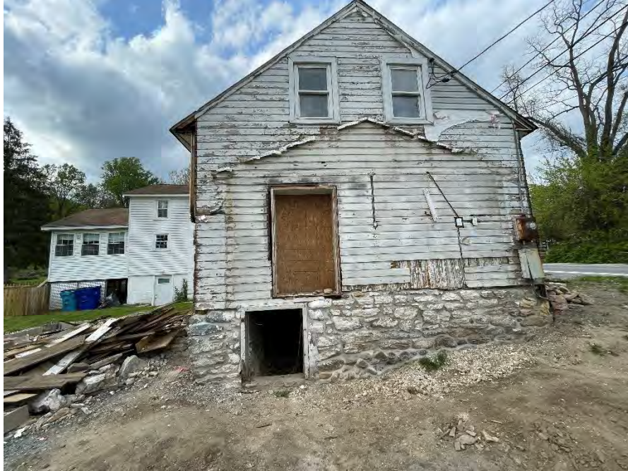
Figure 42: South elevation of the dwelling post-excavation, showing the outline where the south addition was once located, the cased opening connecting it to the original structure, and the entrance to the crawl space beneath it, which used to be in the south addition cellar. Excavation has revealed much more of the original stone foundation, as well as remnants of the previous wood Dutch lap siding and original vertical board siding right of the cased opening. (25 April 2024).
