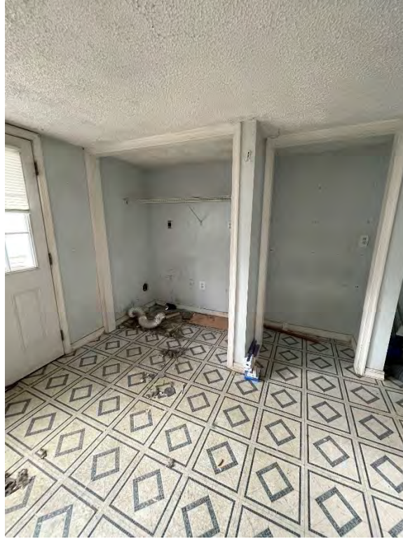
Figure 40: The two closets on the south addition's west elevation. The left one was once the laundry closet.
