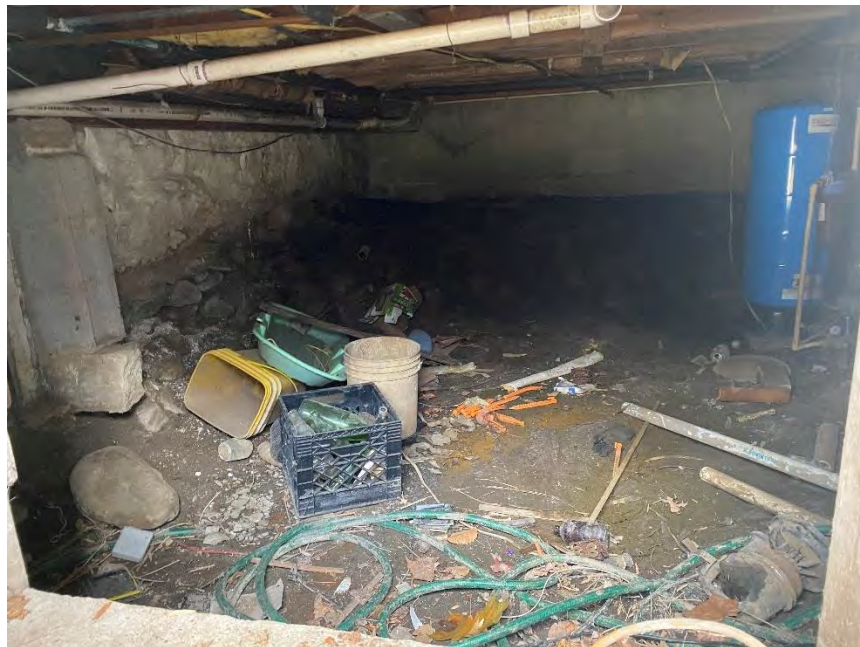
Figure 41: Shallow cellar area beneath the south addition, with a view of the CMU foundation wall and the north original stone foundation left of it. The dwelling's water tank is visible to the right. The moisture seeping out of the earthen floor of the cellar can also be seen, demonstrating the excess groundwater in the area.
