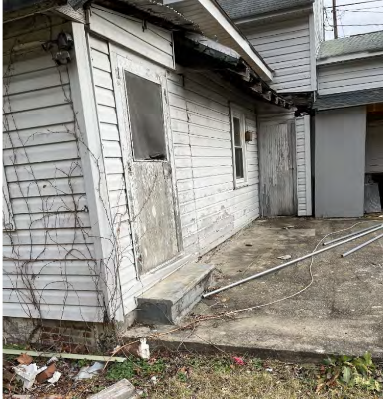
Figure 12: South elevation of the west addition, displaying the concrete patio, the screen door exiting the anteroom, the south-facing summer kitchen window, and the outside tool closet. At the far right of the image is a partial view of the lean-to structure covering the shallow entrance to the crawl space area. The south elevation's wood Dutch lap siding is also visible.
