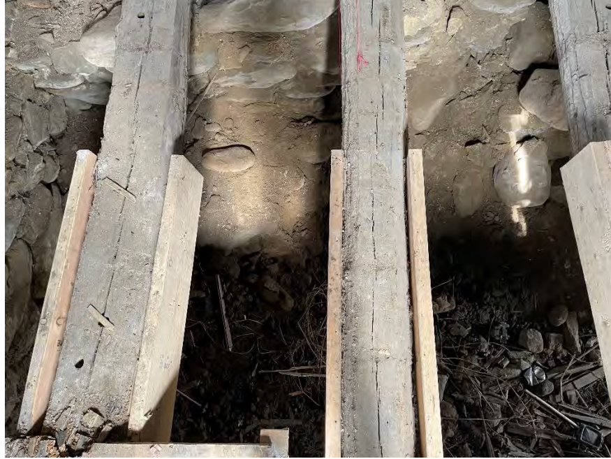
Figure 28: Nonoriginal wood support blocks attached to the original log floor joists on the west elevation of the main dwelling structure. (25 April 2024).
