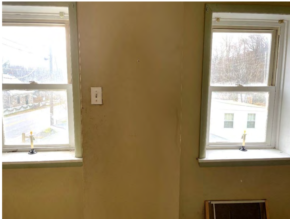
Figure 23: Bump out on the second floor and its position between the two south-facing upstairs windows.
