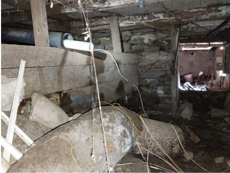
Figure 74: South elevation of the crawl space, providing a much more direct view of the stone hearth base before excavation. Without being able to look at it from above or the eastern portion of the crawl space, there was little to suggest it was anything other than part of the original foundation. There are also nonoriginal floor supports made of wood boards. (11 August 2023). Image courtesy of David Bittle.
