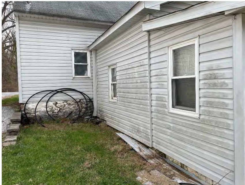
Figure 11: North elevation of the Hoke dwelling west addition and its connection with the main structure, including the corner restroom window along with the north-facing summer kitchen and anteroom windows. The vinyl siding of each exterior wall in frame can be seen.
