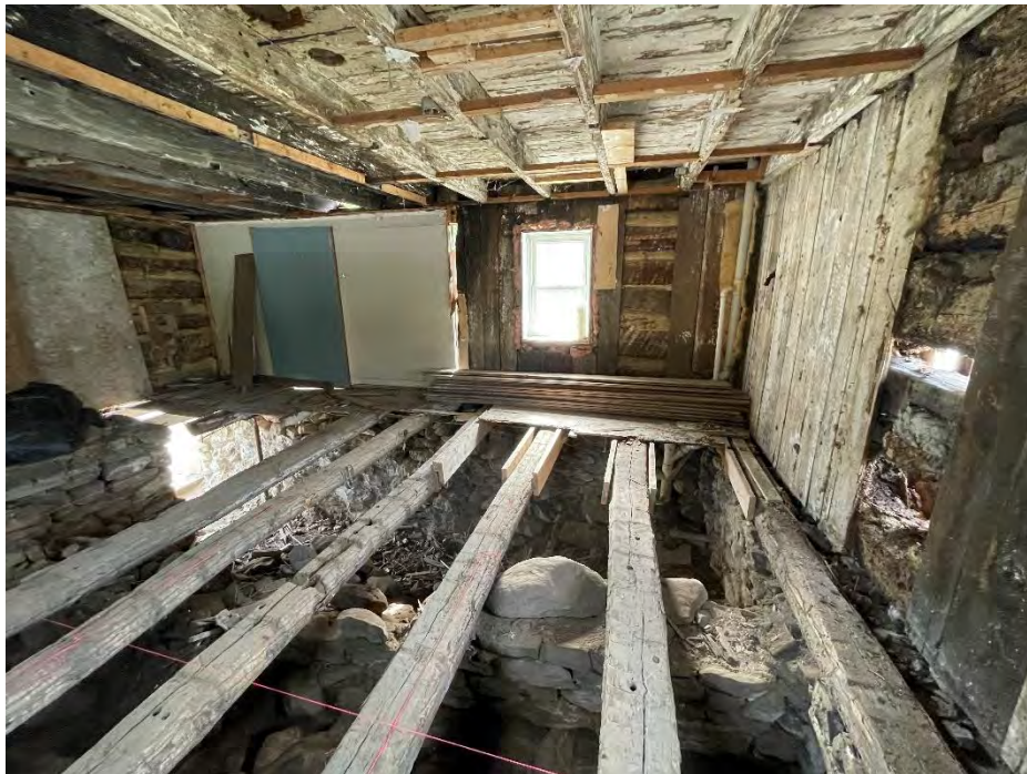
Figure 27: Post-excitation living room from the northeast elevation, showing the small section of nonoriginal flooring left along the west elevation after excavation; the section of drywall that once connected to the west addition; the original log floor joists, walls, and ceiling beams; some of the nonoriginal wood support blocks; and the stone hearth base (far left). (25 April 2024).
