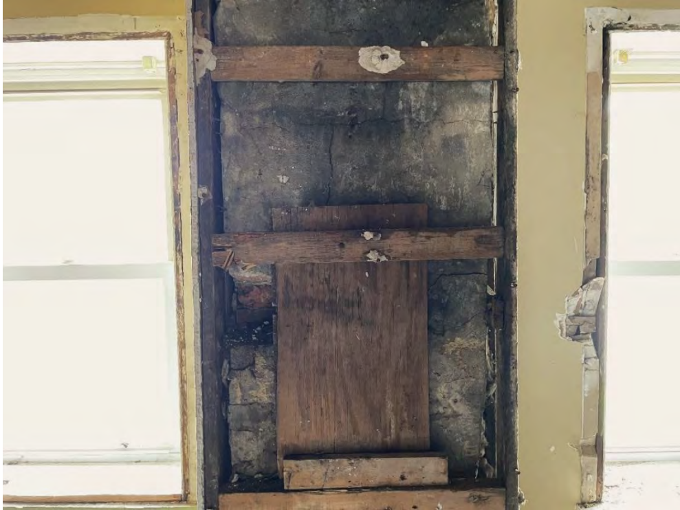
Figure 70: Remains of the chimney stack behind the second-story bump out, supported by wood boards. (25 April 2024).
