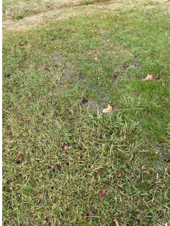
Figure 56: Inundated ground in the Hoke rear yard before any of the excavations or repairs in 2024.
