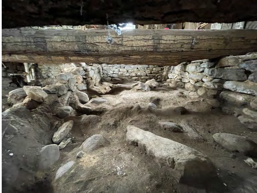
Figure 26: Eastern section of the crawl space area post-excitation, showing the area filled in with stone and earth, as well as the stone wall on the left, which blocked it from access prior to excavation. (25 April 2024).
