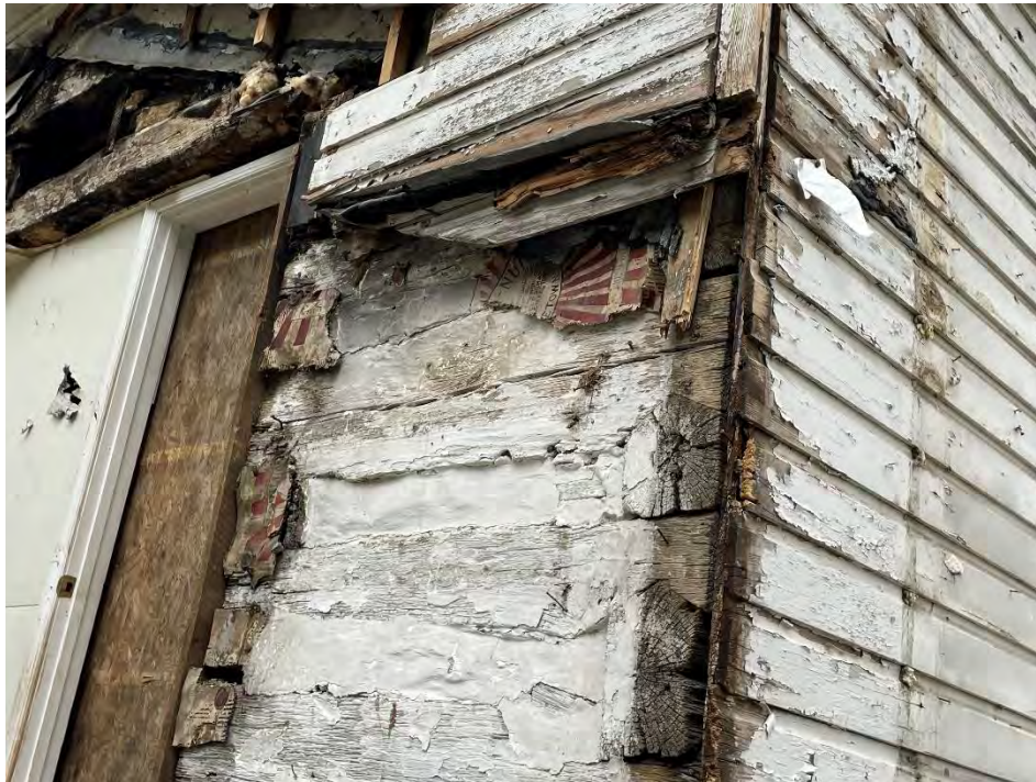
Figure 31: Exterior remnants of poster paper used as insulation attached to the original log wall in the southwest corner of the dwelling, where the outdoor tool closet once was. (25 April 2024).
