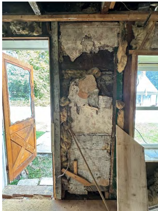
Figure 87: East elevation interior wall between the front door and the southernmost front window post-excavation. Much of the original horizontal log construction is obscured by wallpaper. (10 September 2024). Image courtesy of Elizabeth Comer.
