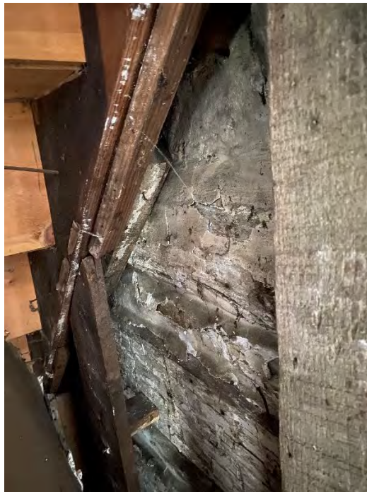
Figure 21: View inside the spandrel closet, with part of the old interior wall visible.
