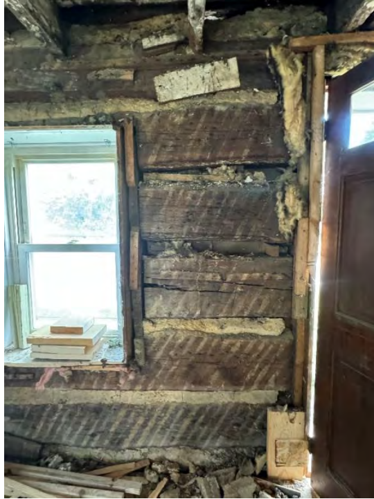
Figure 86: East elevation interior wall between the northernmost front window and the front door post-excavation. Small planks and blocks of wood can be seen intermittently attached to the original log wall. The chinking around the third highest log appears to have deteriorated or otherwise been stripped away, leaving gaps between the logs above and below it. (10 September 2024). Image courtesy of Elizabeth Comer.
