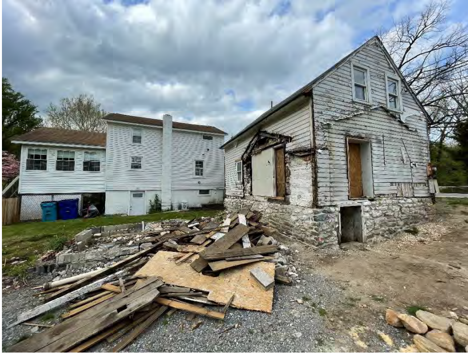
Figure 48: West and south elevations of the dwelling post-excavation. The outlines of both additions are visible on the original dwelling, and much of its original stone foundation has been revealed. The large divot in the ground where the patio and additions all were is evident when compared to pre-excavation photographs. (25 April 2024).
