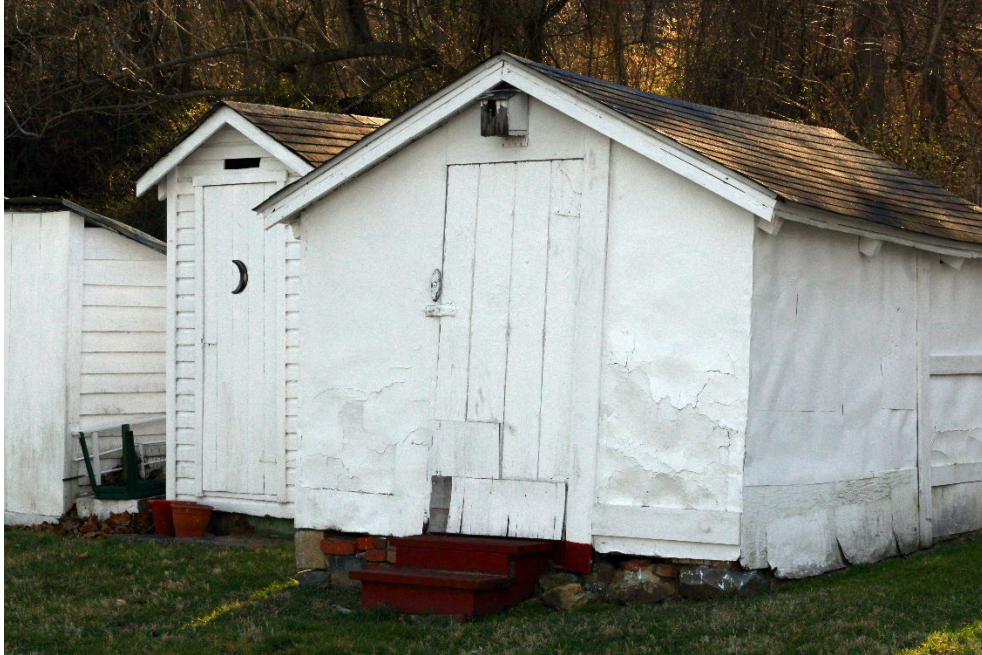
Figure 32: Close-up of the hog pen (front) and the outhouse to the left of it, as well as the chicken coop slightly in view all the way to the left. The roof of each outbuilding can be distinguished, as can the damage to the hog pen and outhouse. The bluebird house mounted above the hog pen door can also be seen with its chipped white paint.
