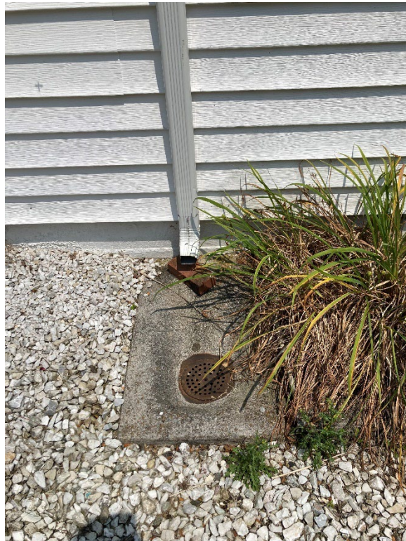
Figure 51: The drain on the west elevation of the dwelling which directs water from the gutters into the underground pipe system connected to the underground stream. (June 28, 2023).
